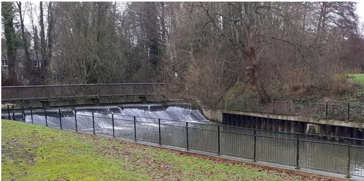
Figure 3. Cedar Close weir. The bypass channel would re-enter the river immediately to the right of the weir.
